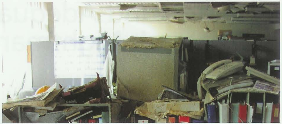
Ceiling collapse damage
